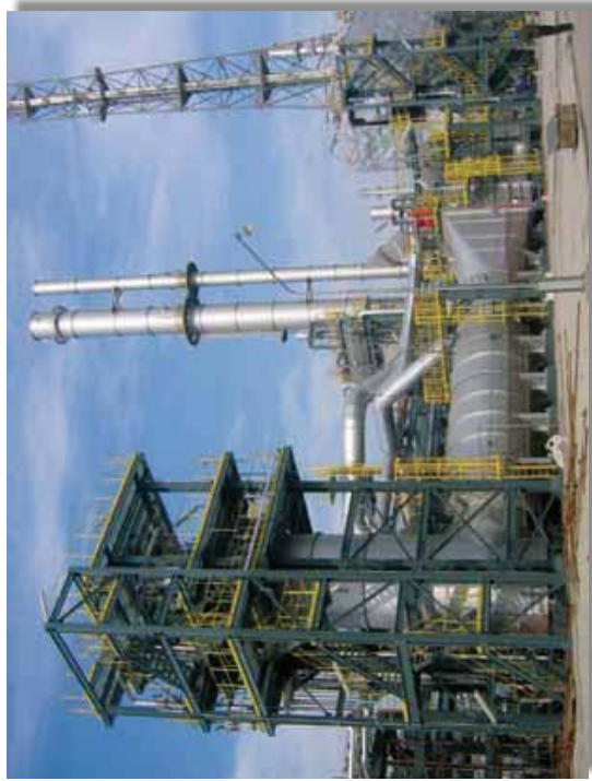
Multi-Stage, Low NOx WasteWater Incinerator supplied to handle 129 MM Btu/hr from an acrylonitrile production facility in Shanghai, China
