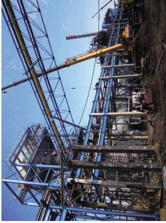
Construction efforts during installation phase of an Acrylonitrile Waste Water Incinerator project in Jilin, China
