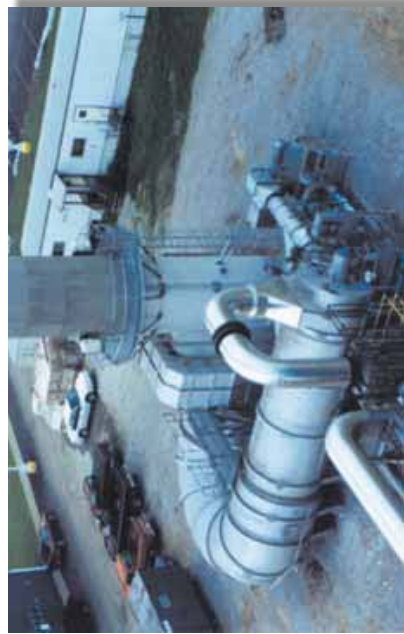
Carbon Black Tail Gas (Two Stage) Thermal Oxidizer 19,237 scfm 96 MM Btu/hr 200 Ft. Free Standing Stack Natural Gas
